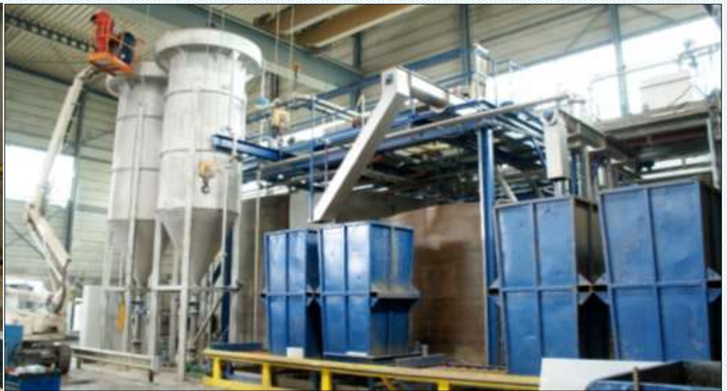
Separators ExSep in production environment (Germany)
