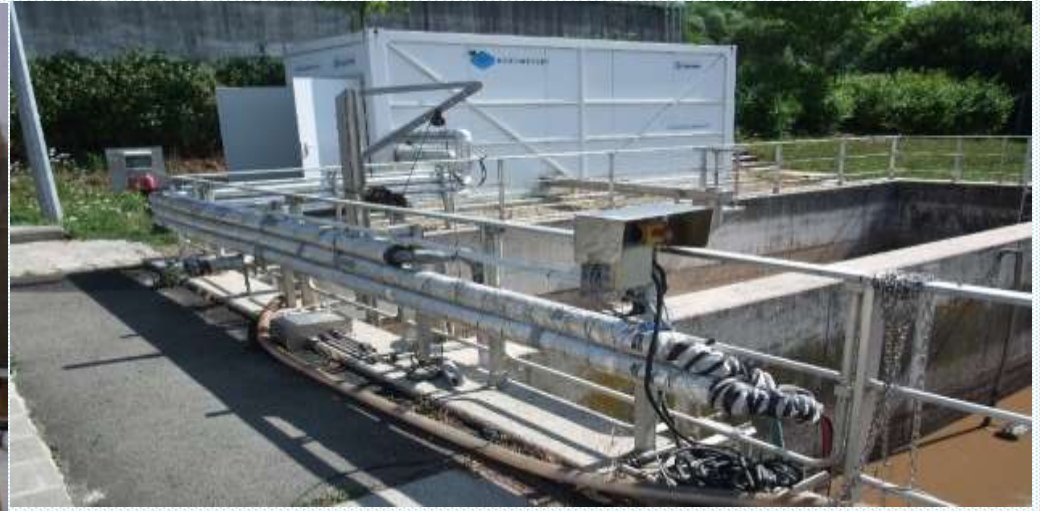
Box4Water-WW in Luxembourg
