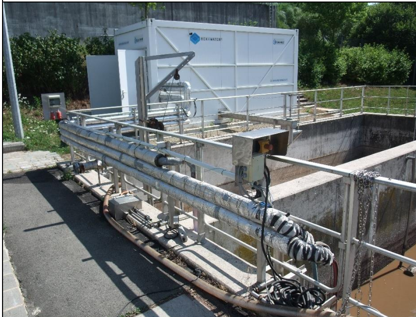
Upgrade in Luxembourg using a containerized system
