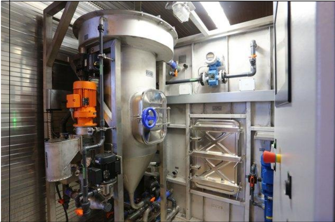
View inside Box4Water with ExSep® for pre-treatment
